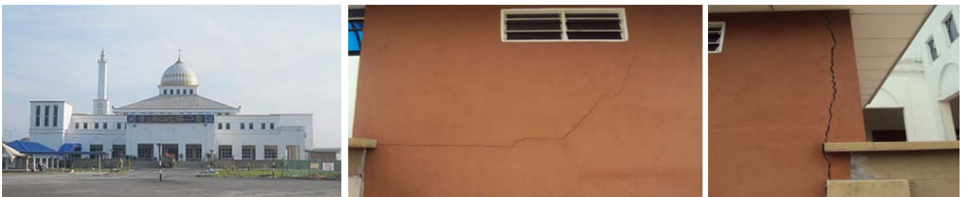
Figure 1: Cracks on building wall in Masjid Seri Ampangan, Nibong Tebal, Pulau Pinang
