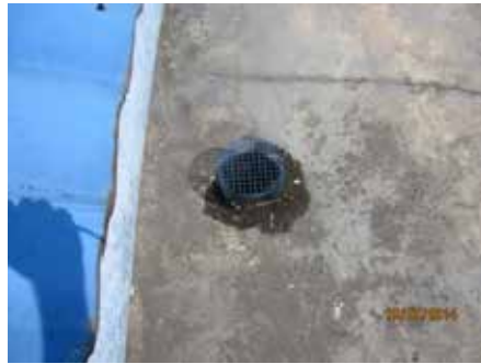
Figure 4: Condition of RWDP 2
