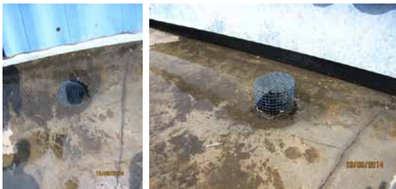
Figure 15: Inefficient flow of water due to the presence of dirt around RWDP 2
