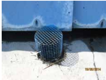
Figure 7: Condition of RWDP 5
