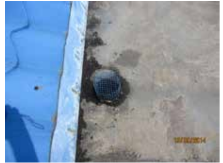
Figure 5: Condition of RWDP 3
