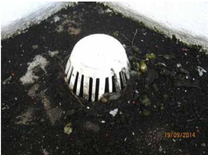
Figure 11: Condition of RWDP 9
