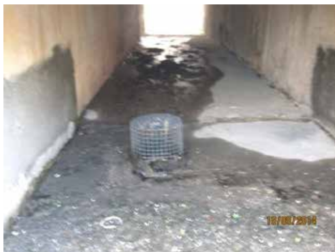
Figure 14: Condition of RWDP 12
