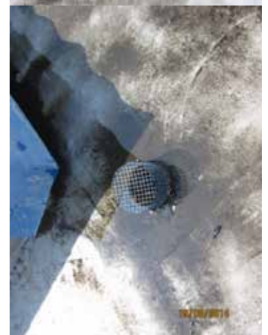
Figure 10: Condition of flat roof surface near RWDP 8 showing the existence of water ponding
