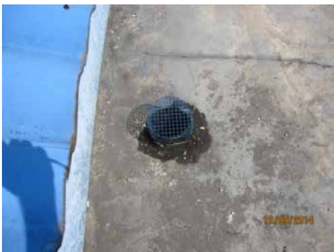
Figure 13: Condition of RWDP 11
