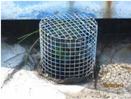
Figure 3: Condition of RWDP 1
