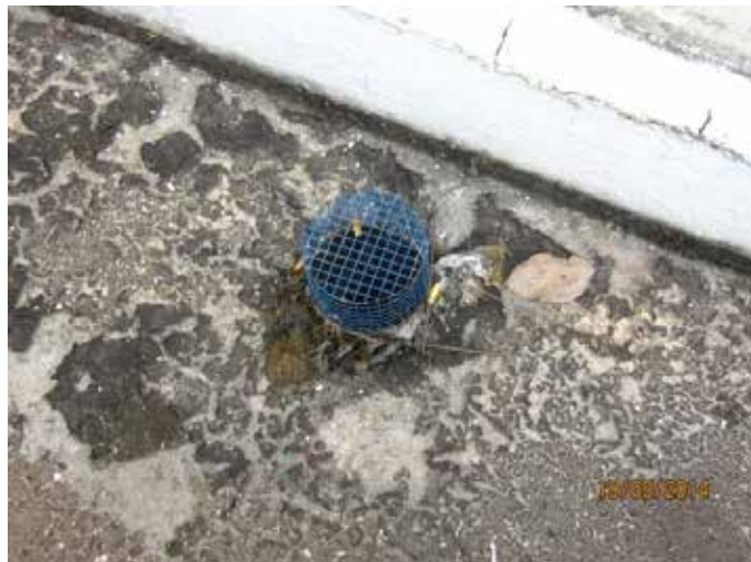
Figure 12: Condition of RWDP 10
